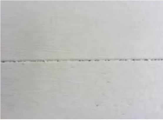
Post application inspection shows sheathing joint not properly sealed. Reseal with sealant.
